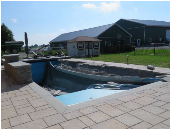
Fiberglass pool collapsed under imbalanced lateral pressures (Photo credit: Y Korany)
