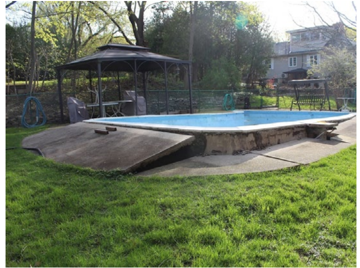
Concrete pool pushed out of ground by hydrostatic pressure (Photo credit: AJ Lohonyai)
